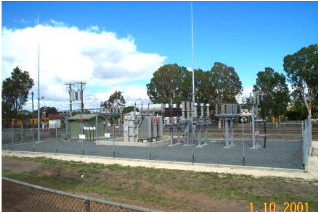
Ergon Energy 10MVA 66/11kV Substation installed in 2000 to increase export capacity to 10MW
